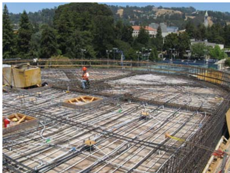
Fig. 3: Although much of the mechanical and electrical systems were located under a raised floor (instead of hanging from the ceiling), the floor slabs contained lighting conduit and tubing for the hydronic heating and cooling system in addition to the prestressed and mild reinforcement
