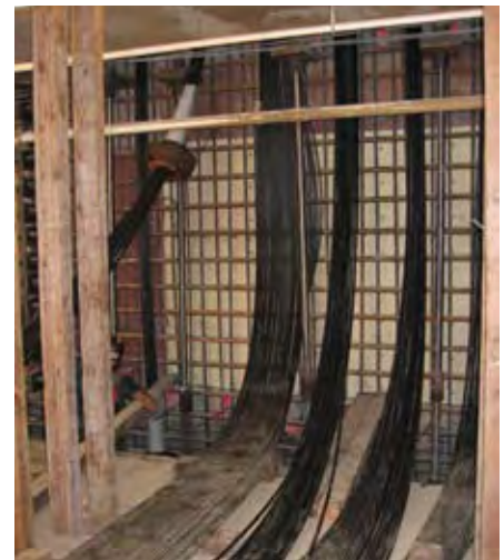
Fig. 6: Due to equipment constraints in the building, each strand for the bundled tendons was individually installed through the floor opening cut in the floor slabs
