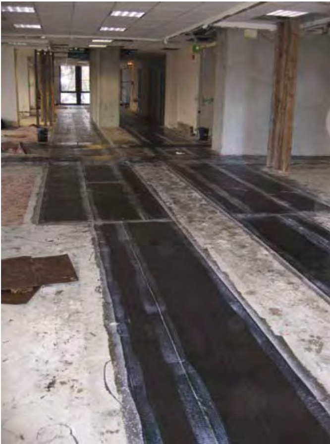
Fig. 10: Carbon fiber collector elements installed on the floor slab and later concealed under the floor covering
