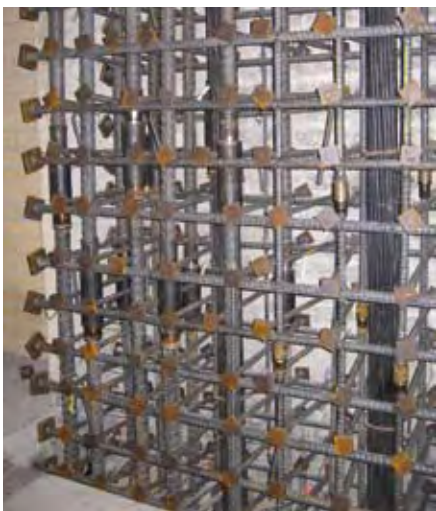
Fig. 8: Boundary element region of shearwall showing mechanically spliced No. 18 (No. 57) vertical bars, headed shear and cross-tie reinforcement, and post-tensioning tendon
